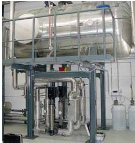
Pre-assembled feedwater pumps and tanks
