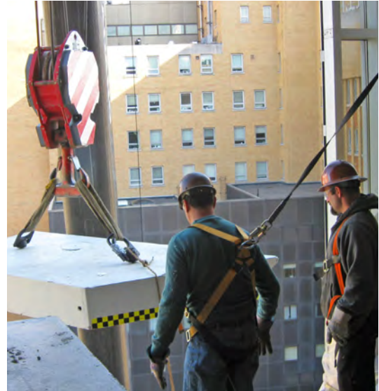
View from the top: Installation crew members keep a close eye on the crane while it lowers a concrete slab into the cyclotron facility on the 9 th floor.
