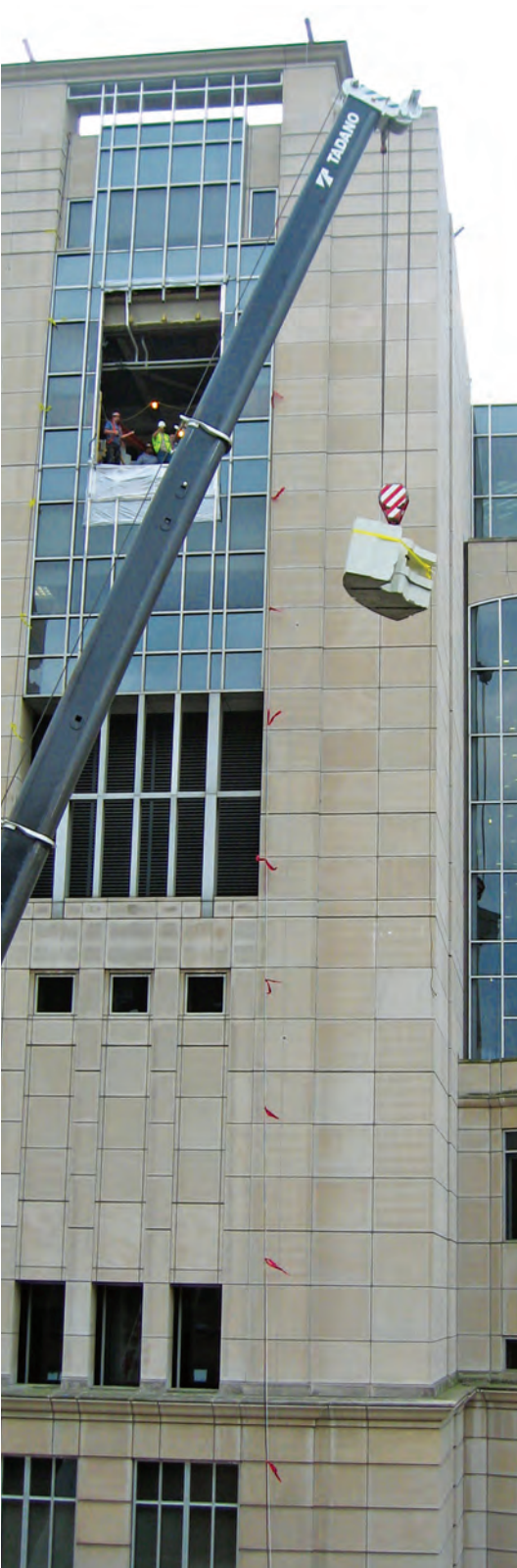
View from the ground: A special crane—only one of the two in existence in the United States—hoists a major piece of the cyclotron shielding onto the 9 th floor.
